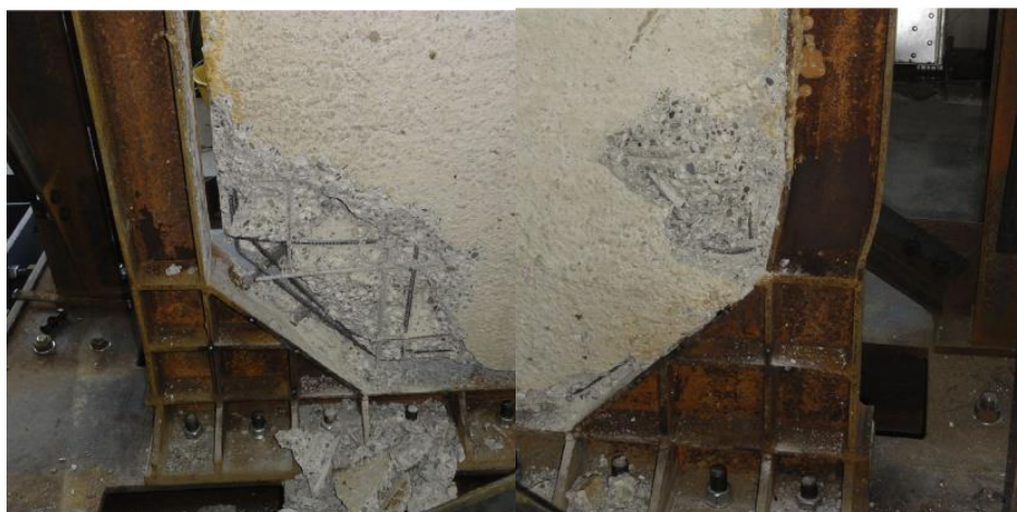
Fig. 5. Failure mode of SRCW specimen
